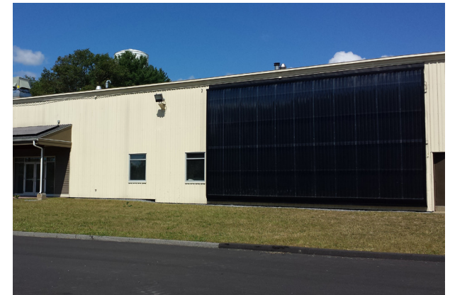
This solar heat reduces the amount of fuel used for space heating.
